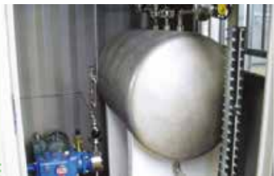
Odorant injection equipment
