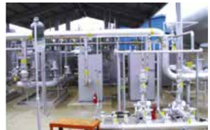
LPG vaporization and mixed equipment
