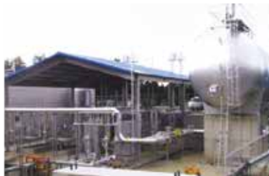
Mixed gas supply equipment
