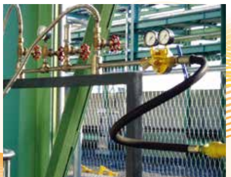
N 2 Purge system
