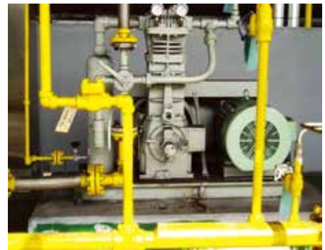
Ammonia unloading compressor
