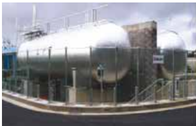
LPG storage facilities
