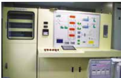
Main control room
