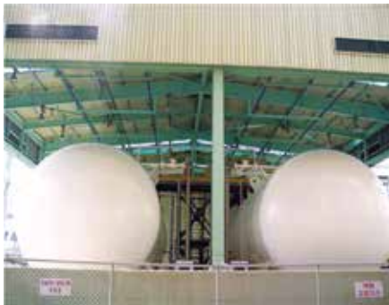
Ammonia storage tank
