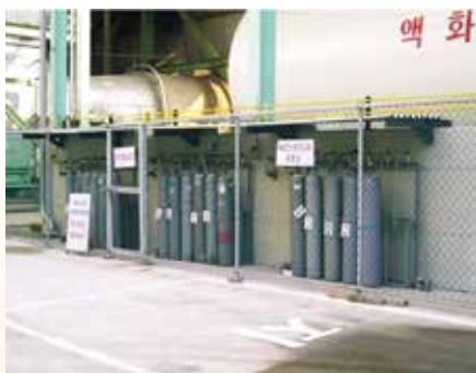
N 2 Purge system
