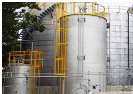
Aqueous ammonia storage tank
