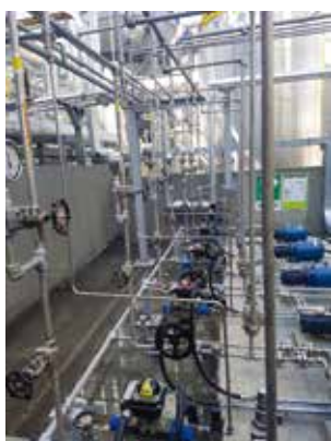
Aqueous ammonia supply system
