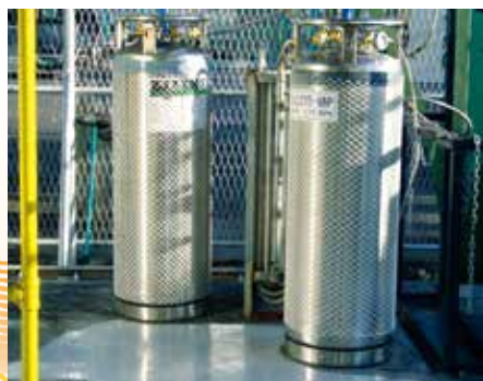
N 2 Purge system
